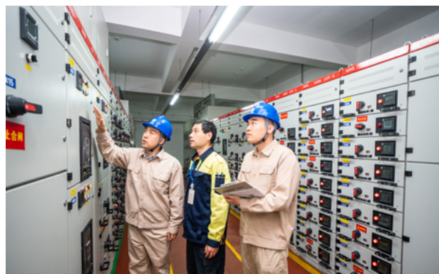
Employees from State Grid Wuxi inspect the power equipment of the park.
