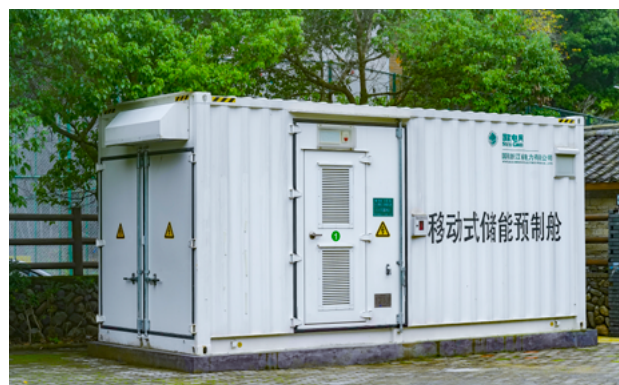
A mobile prefabricated energy storage cabin in Dajun Town
