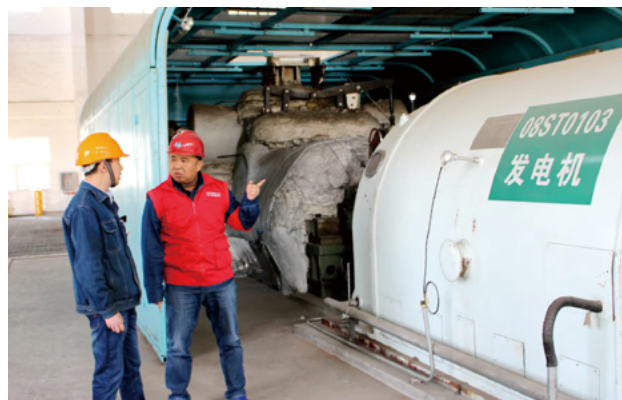
Power supply employees conduct on-site inspections at Ningxia Hening Chemical Co., Ltd. to inspect the electricity substitution.
