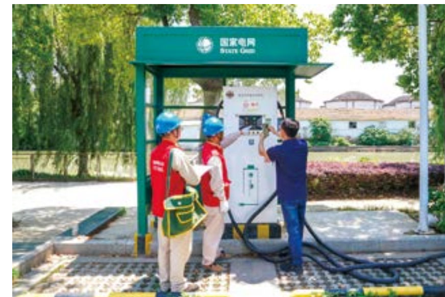
The workers of State Grid Kunshan Power Supply Company carry out safe electricity inspection for the charging piles
