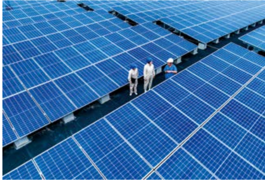
The workers of State Grid Kunshan Power Supply Company check the dust on the roof photovoltaic panel of an enterprise
