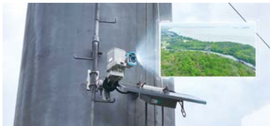
A video surveillance device mounted on a power transmission tower in Wuxi waters
